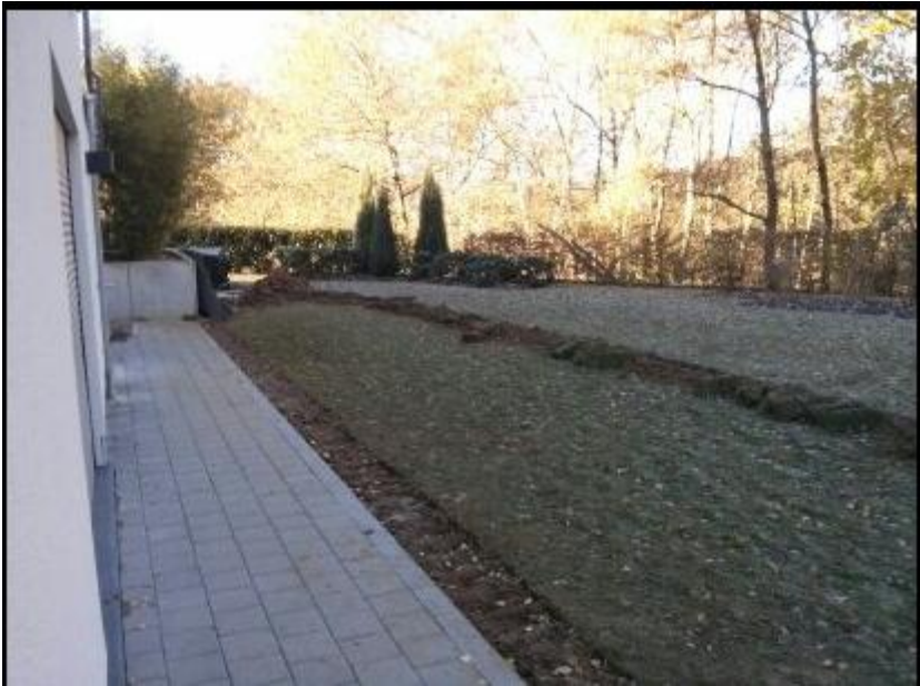
Digging a trench in the courtyard – before the installation of our SafeWay systems.
